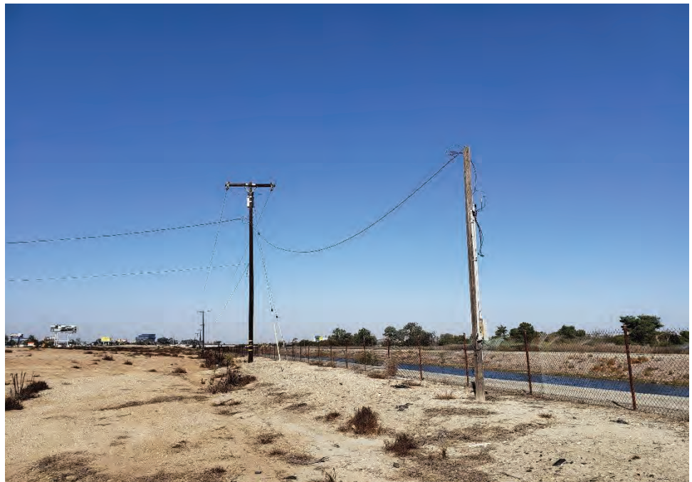
Photograph 12: View of pole-mounted transformer on the eastern portion of the site.
